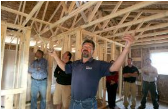
Lance Schmidt, of F.G. Ayers Inc. talks about the type of trusses used in the roof at the the Home Builders Association and Urban Neighborhood Corp. demonstration house in Akron. (Mike Cardew/Akron Beacon Journal)
